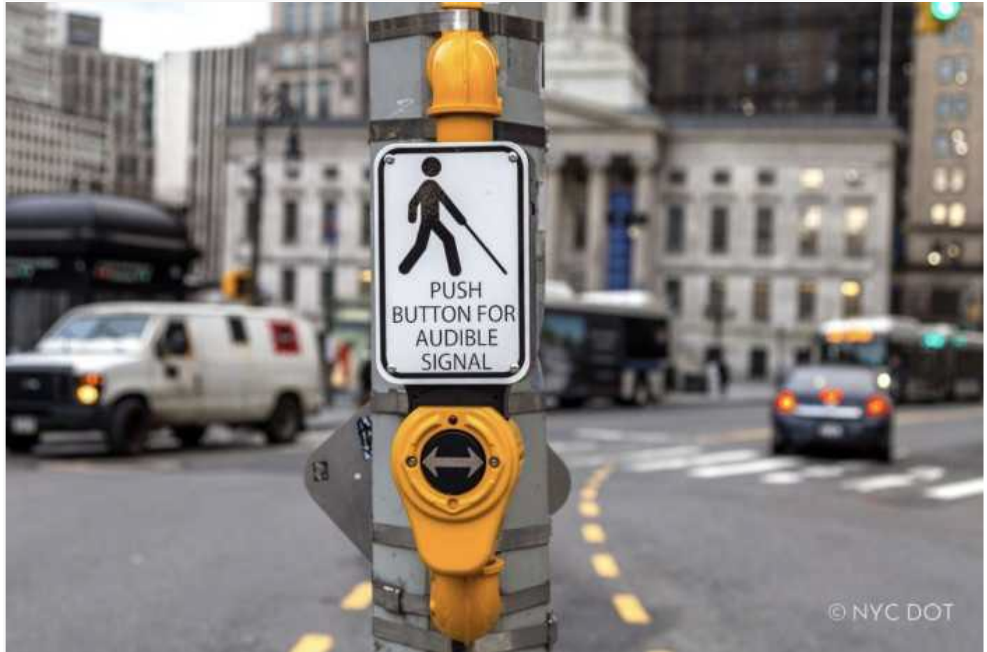
Accessible pedestrian signal (APS) Installed at Court Street in Brooklyn NYC DOT
