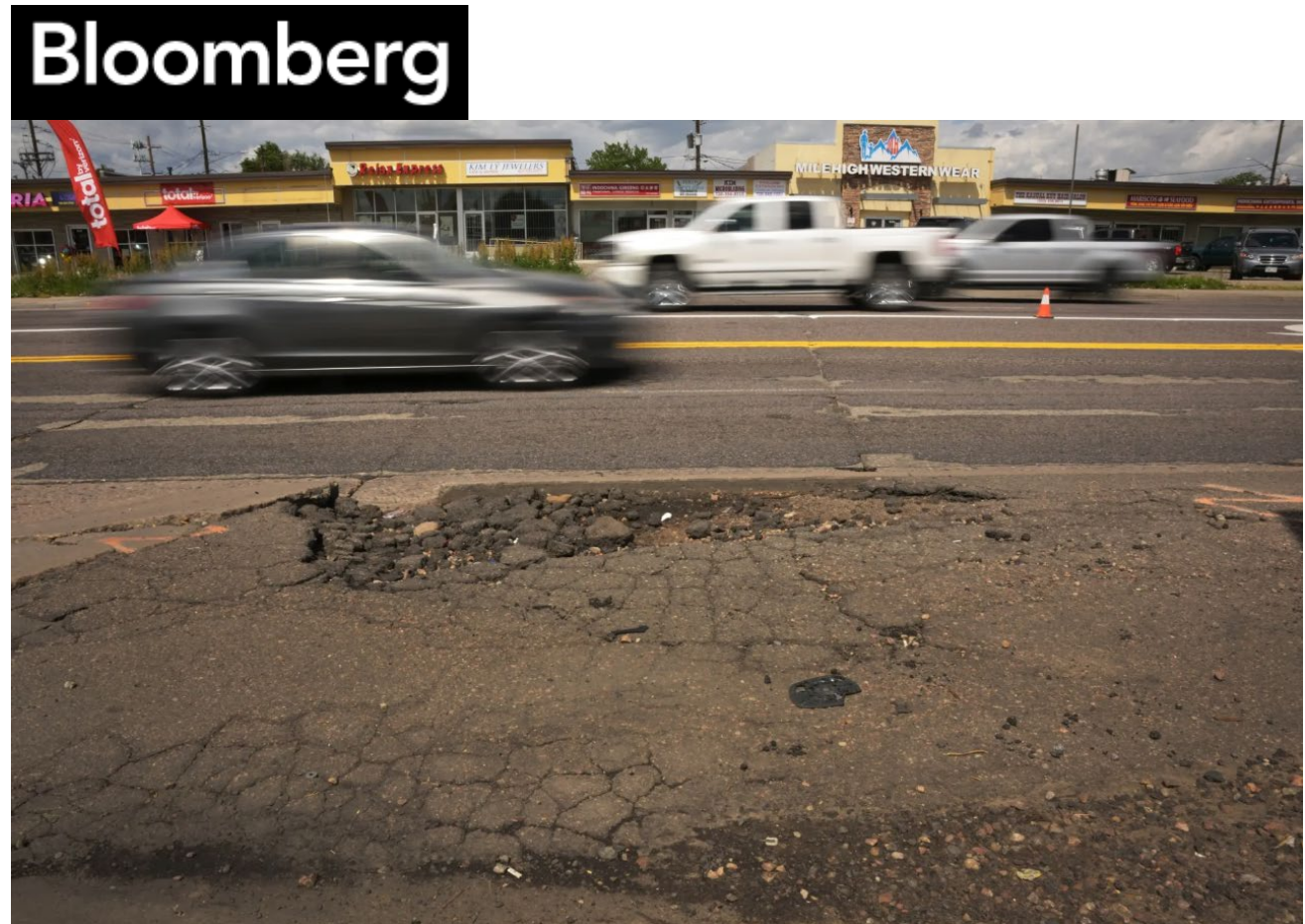
Heavily damaged sidewalks line a roadway in Denver's Little Saigon business district in 2024. A new sidewalk fee for all property owners is set to reform the city's Photographer: Hyoung Chang/Denver Post
