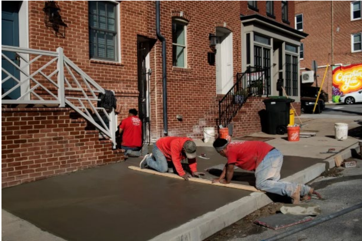
Workers fix a sidewalk in the Baltimore's Canton neighborhood in 2020. Photographer: Brendan Smialowski / AFP via Getty Images
